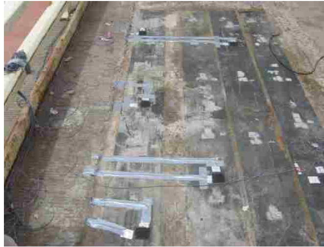
Figure 5-54 All the strain gauges after being installed on the FRP sheets and connected to the wires transmitting the strain signals to the DAQ device.
