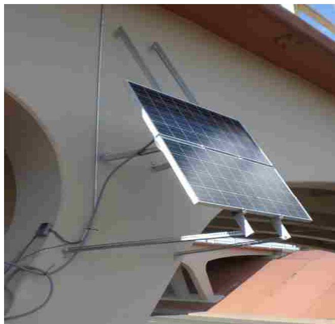
Figure 5-59 Solar power system installed on Bridge 7937 to provide clean renewable energy for the SHM system.
