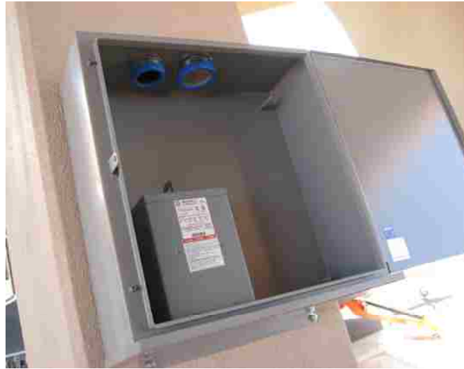
Figure 5-47 Steel box used for housing the data acquisition system and all SHM components.
