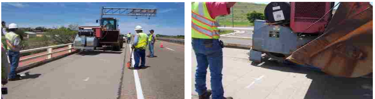
Figure 5-11 Concrete surface milling showing the process of marking the zone and milling.
