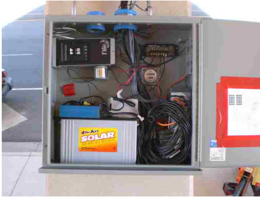
Figure 5-57 Data acquisition system, rechargeable batteries, power inverter, digital timer switch and the wireless modem located at the steel box.
