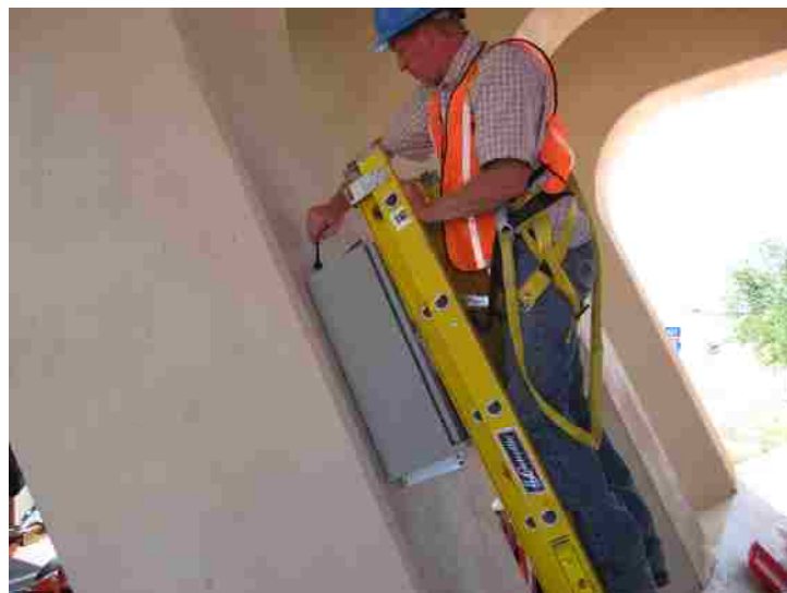
Figure 5-46 Installing of the steel box to house all electrical components at the bottom of Bridge 7937.
